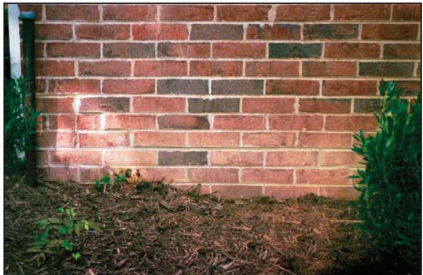
After HELICAL PIER foundation systems stopped the foundation from sinking. Mortar repairs now will have a chance to last, too.
